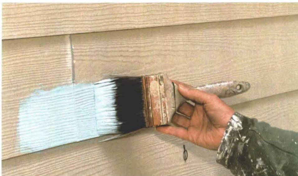
Caulk and paint make expansion gaps disappear. Gaps at plank ends and butt joints must be left for expansion in fiber-cement siding. These gaps are filled with latex caulk, and a coat of paint makes the seams disappear.
